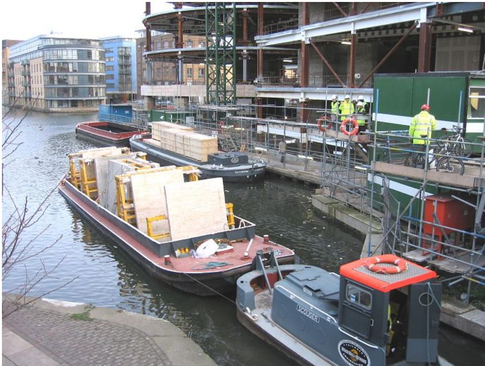
WHH Dutch barge and tug Scouser arriving at Kings Place, London with construction materials. Behind is WHH ex-Leeds and Liverpool short boat Cliithroe (WHH)
