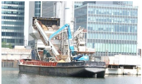
1,000 tonne-plus barge serving floating concrete batching plant at Wood's Wharf, London (D Hilling)
