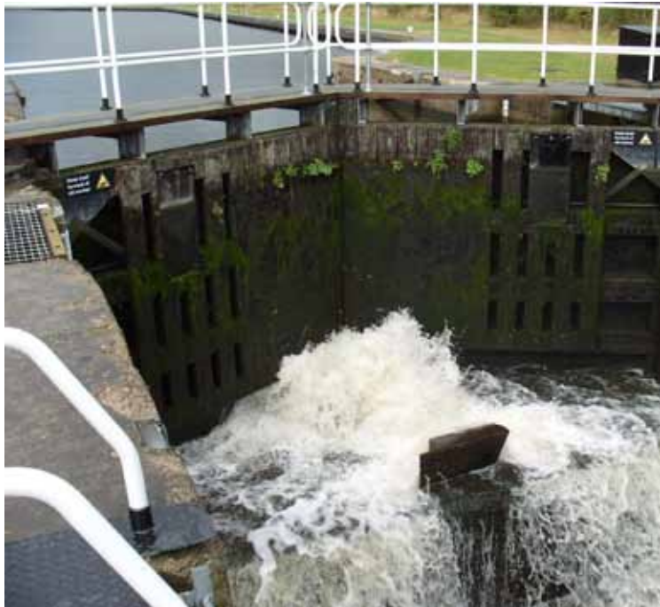
The blown cill at Lemonroyd lock with all the sluices and gates fully closed!
