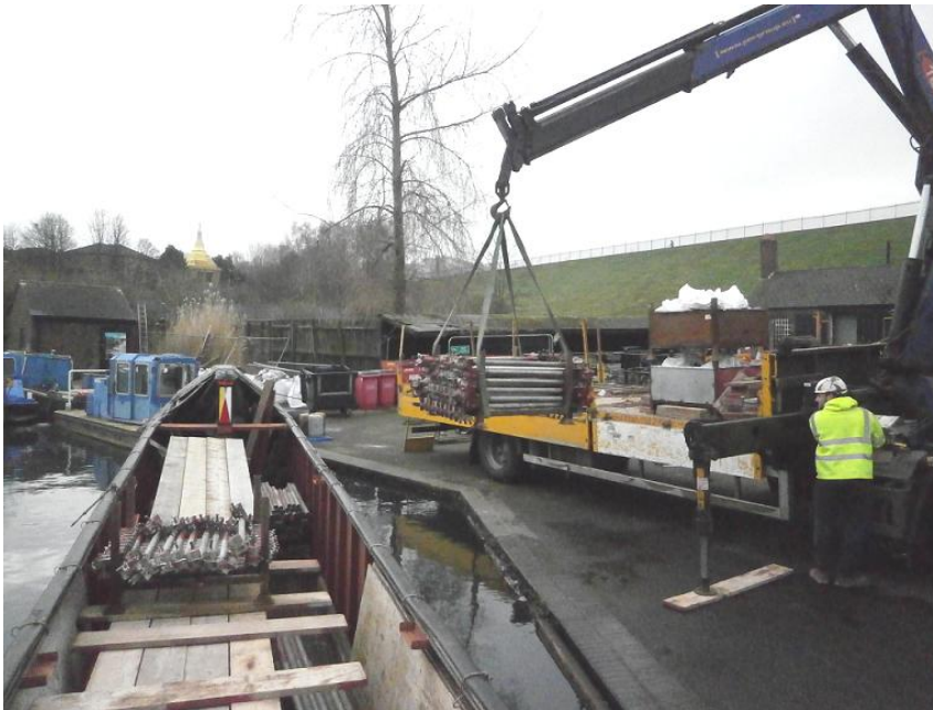
Narrow boat Arundel loading scaffolding at the CRT yard at Icknield Port, Birmingham (R Horne)
